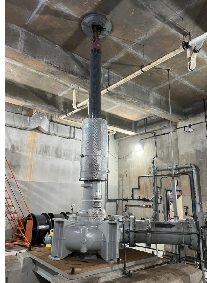
Mauldin Road New Influent Pump and Shaft
