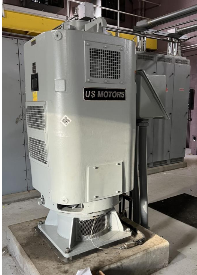
Mauldin Road New Influent Pump Motor
